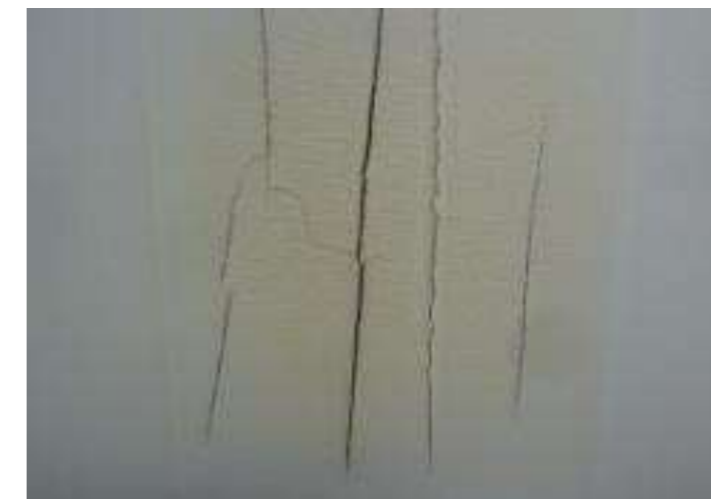
Backsheet deep cracking
